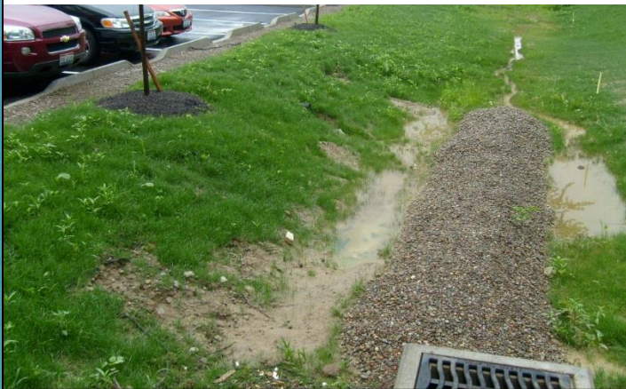
Common setup outside the outlet structure (gravel covering a perforated pipe)
