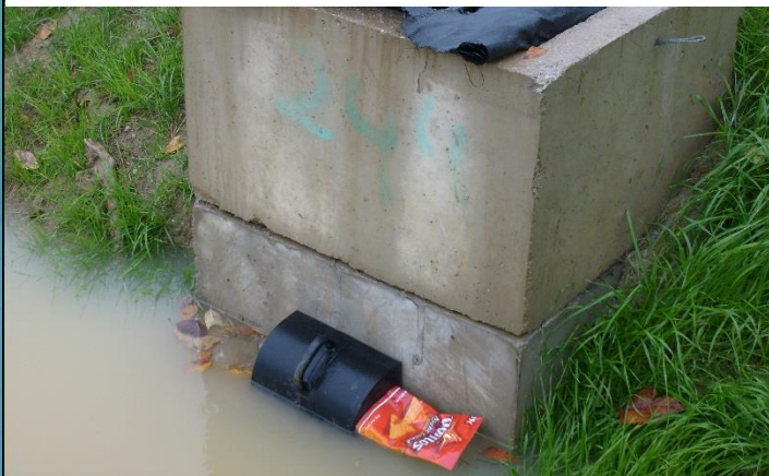
A "hood" protects the small (<3") stage 1 orifice from getting clogged with floating debris
