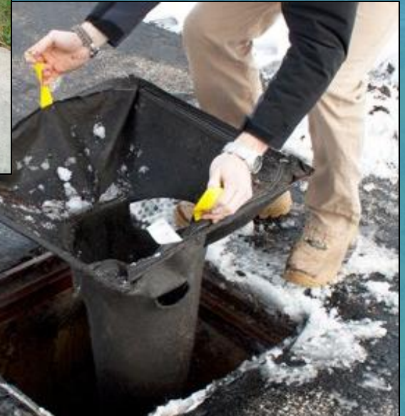
Catch basin inserts are often used on storm sewers that discharge directly into a bioretention cell.
