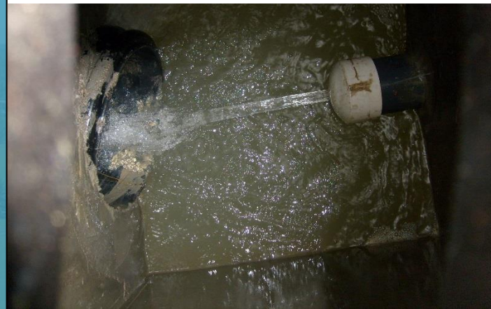
Common setup inside the outlet structure (stage 1 orifice is drilled into the cap on a pipe)
