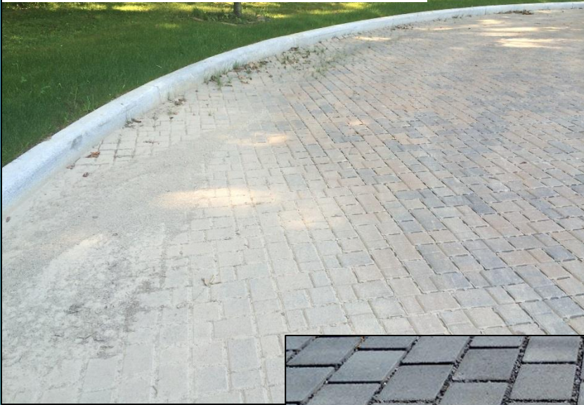
Permeable pavers clogged with sediment
