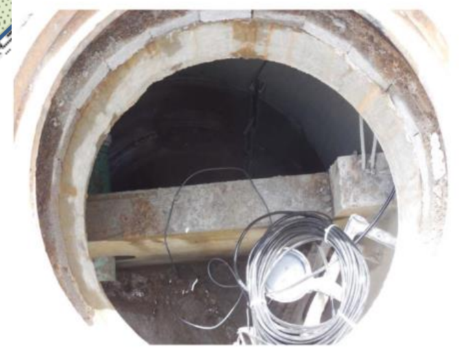
Sensor Installation Photo
