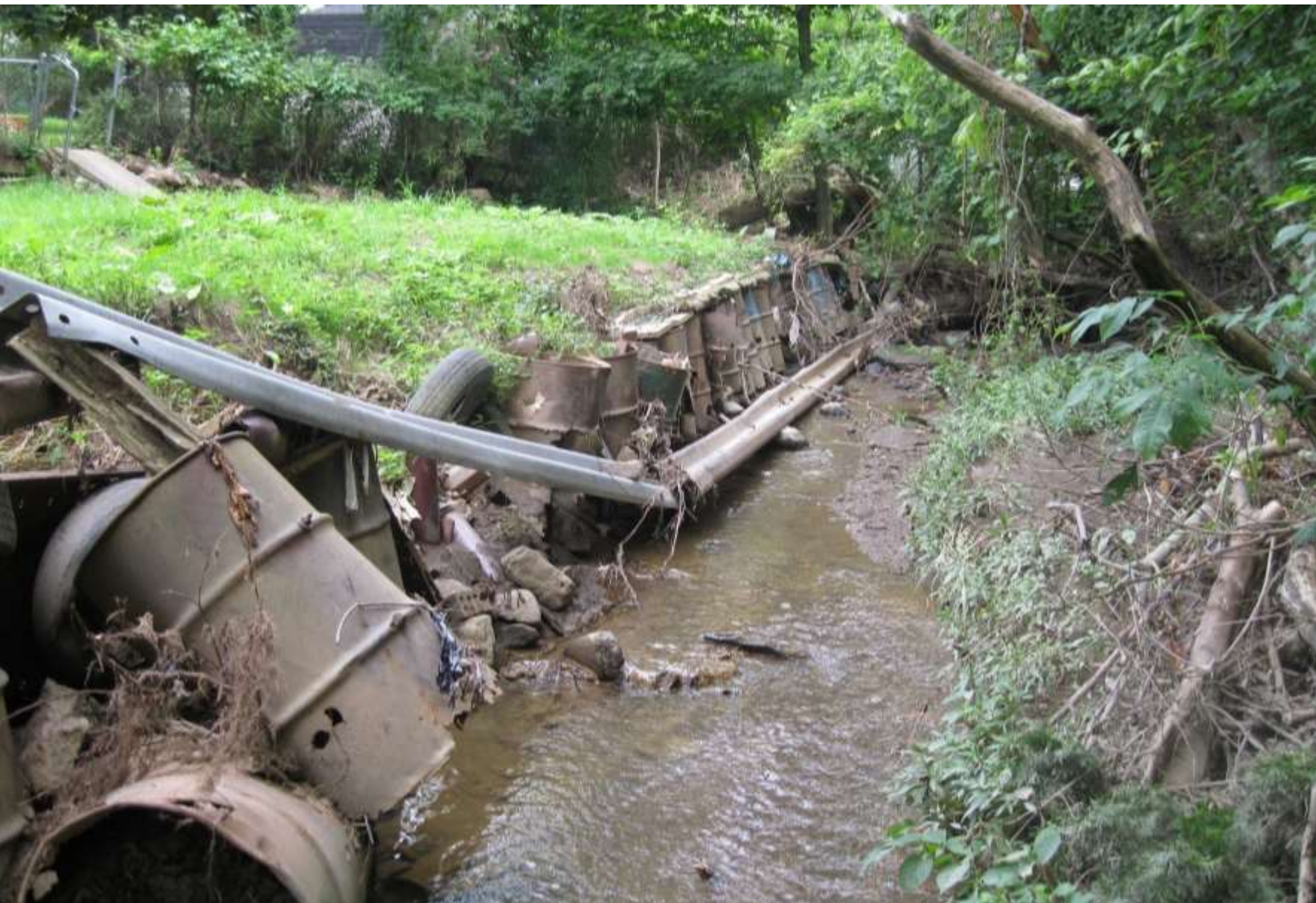
Streambank erosion Baldwin Creek August 2011
