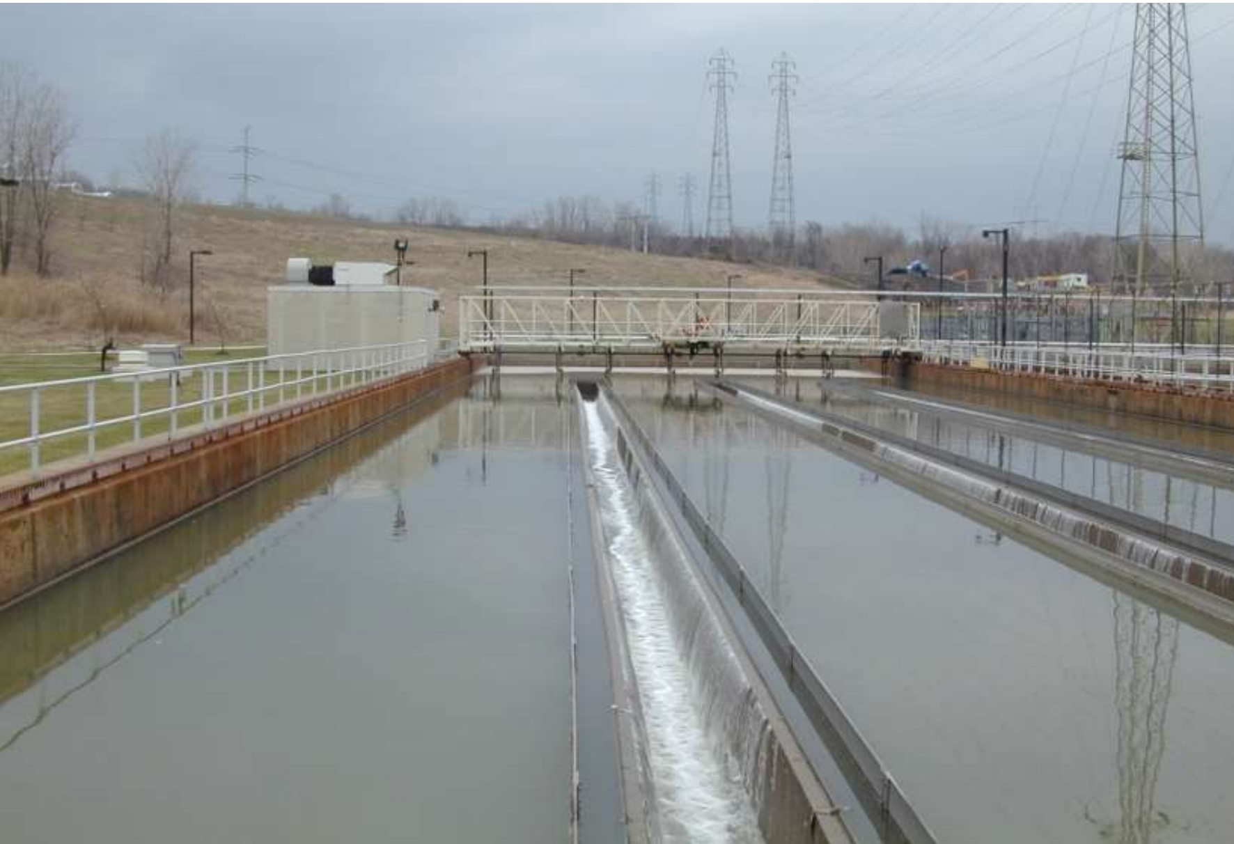
Primary Treatment Primary Settling Tank
