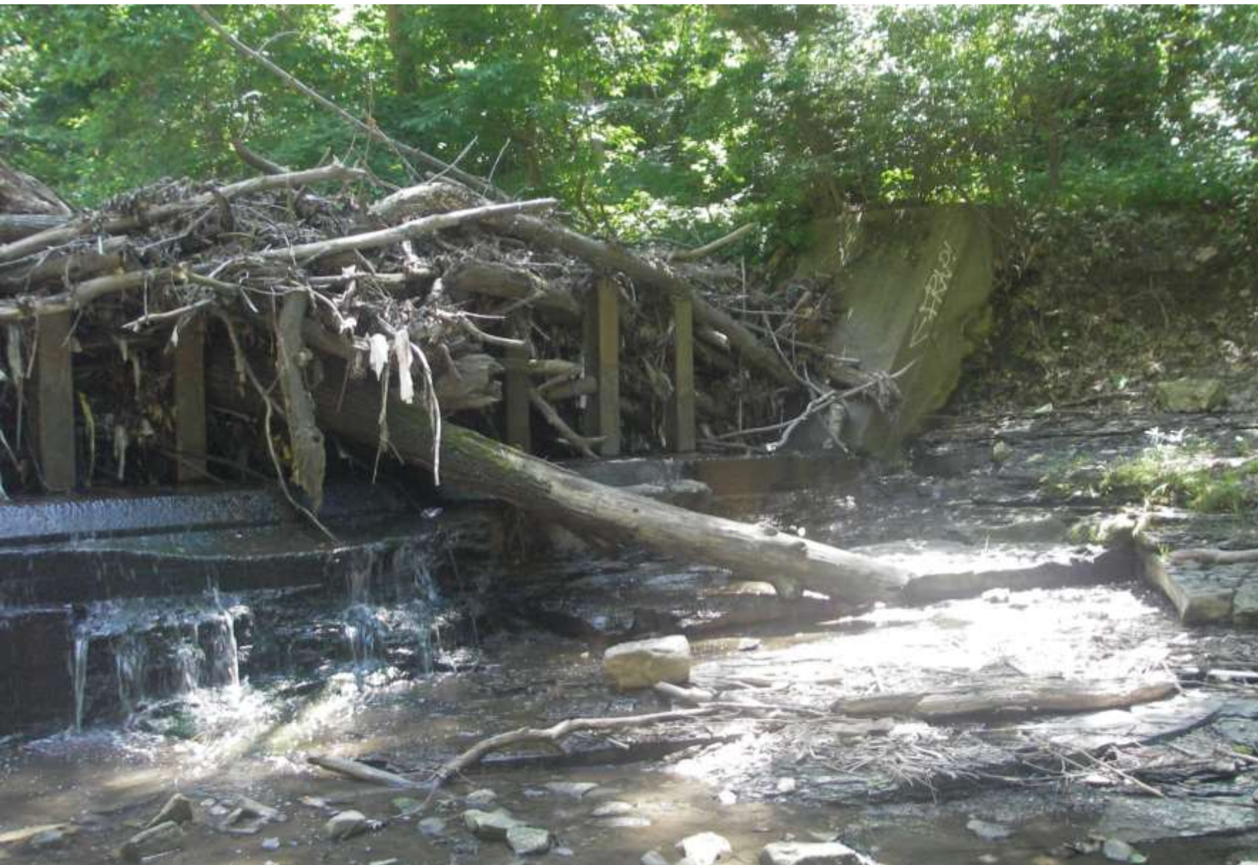
Debris along Dugway Brook Cleveland Hts, Ohio
