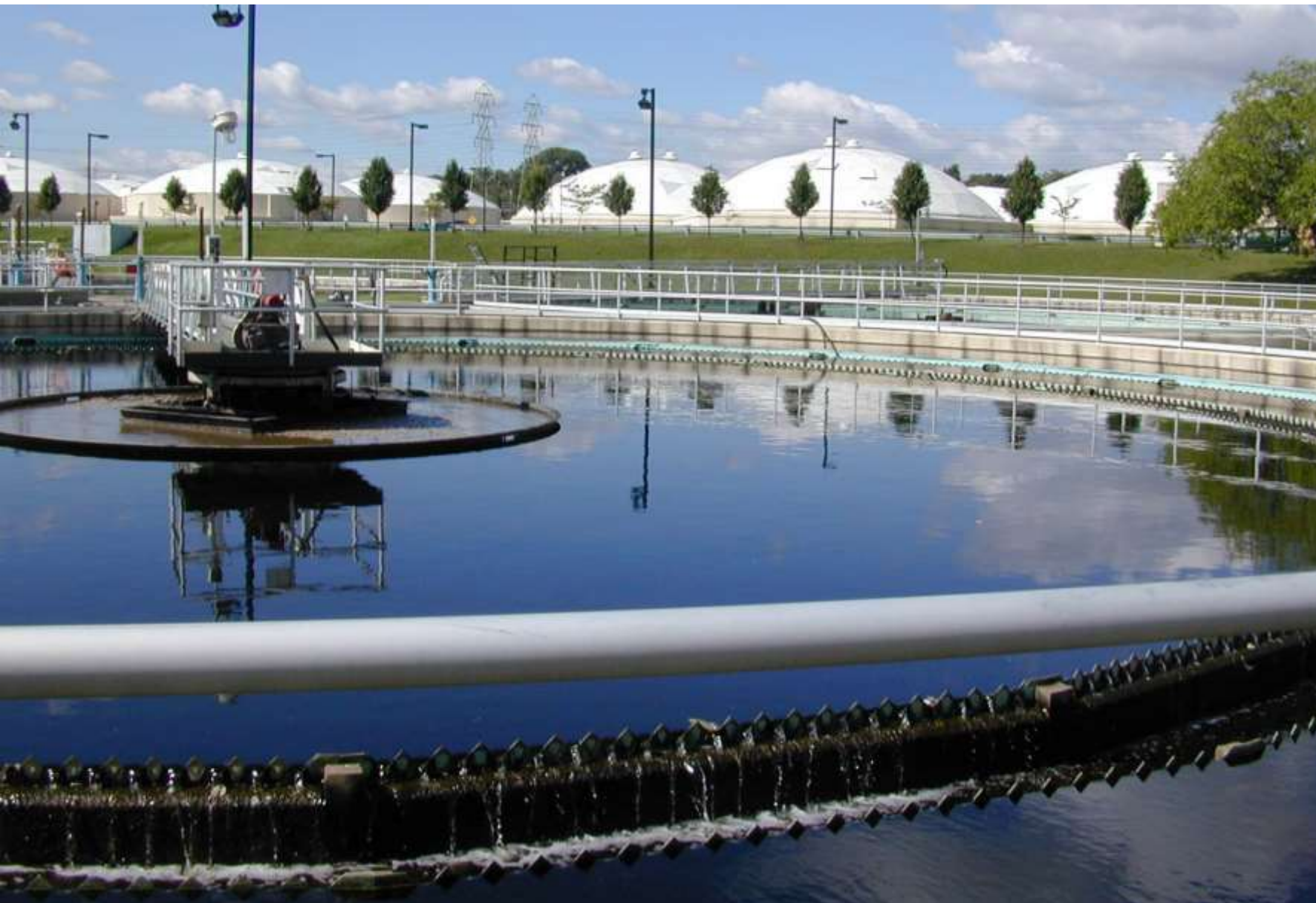
Secondary Treatment Final Settling Tank
