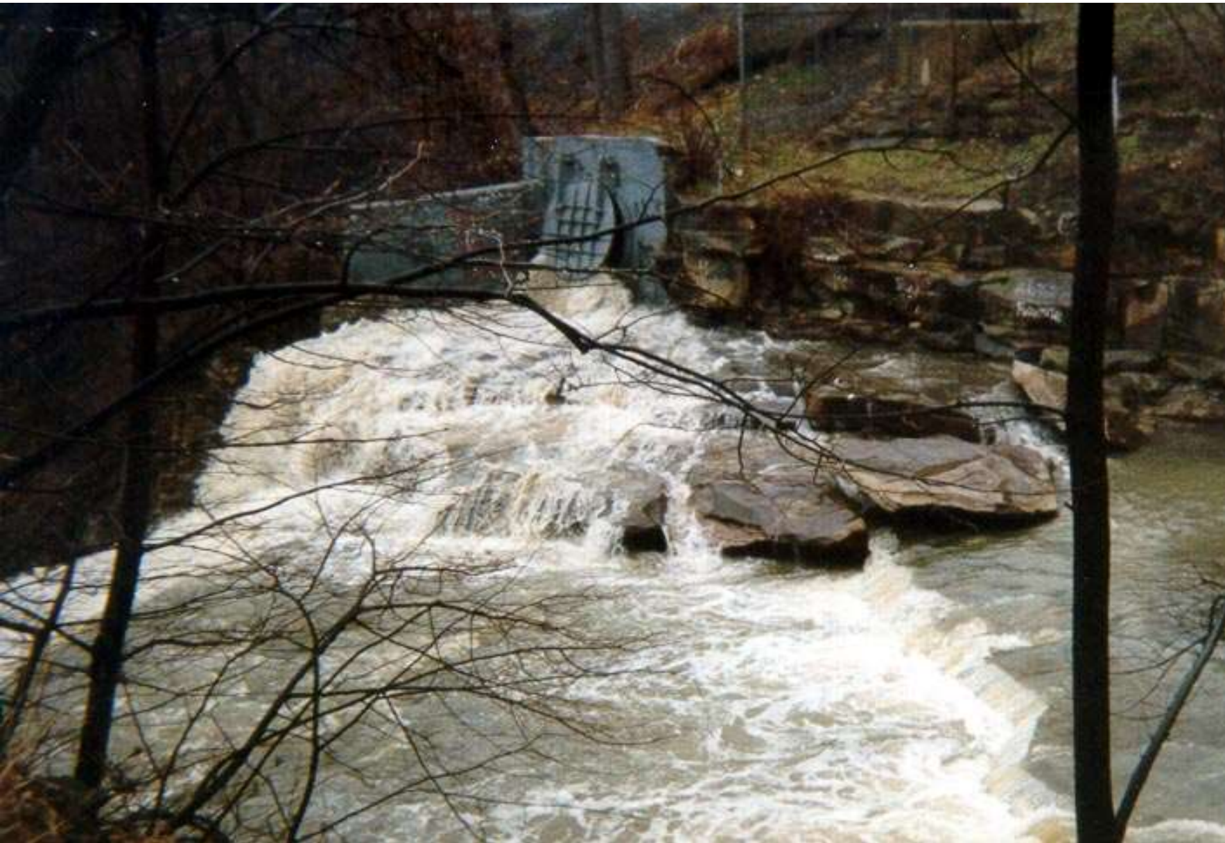
Combined Sewer Overflow (CSO)
