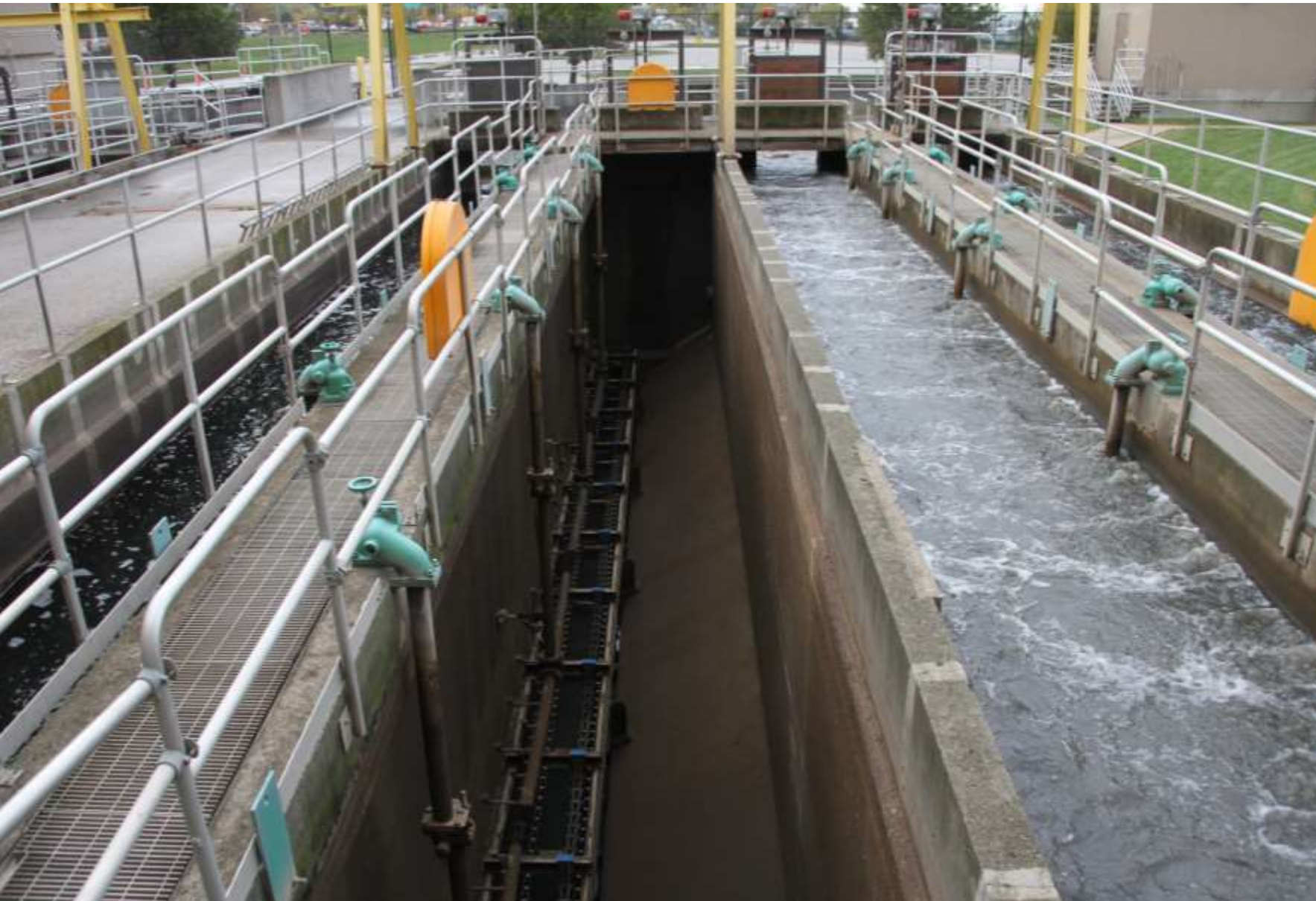
Preliminary Treatment Aerated Grit Channel
