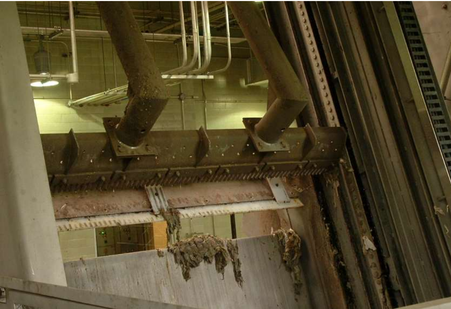
Preliminary Treatment Mechanical Bar Rakes
