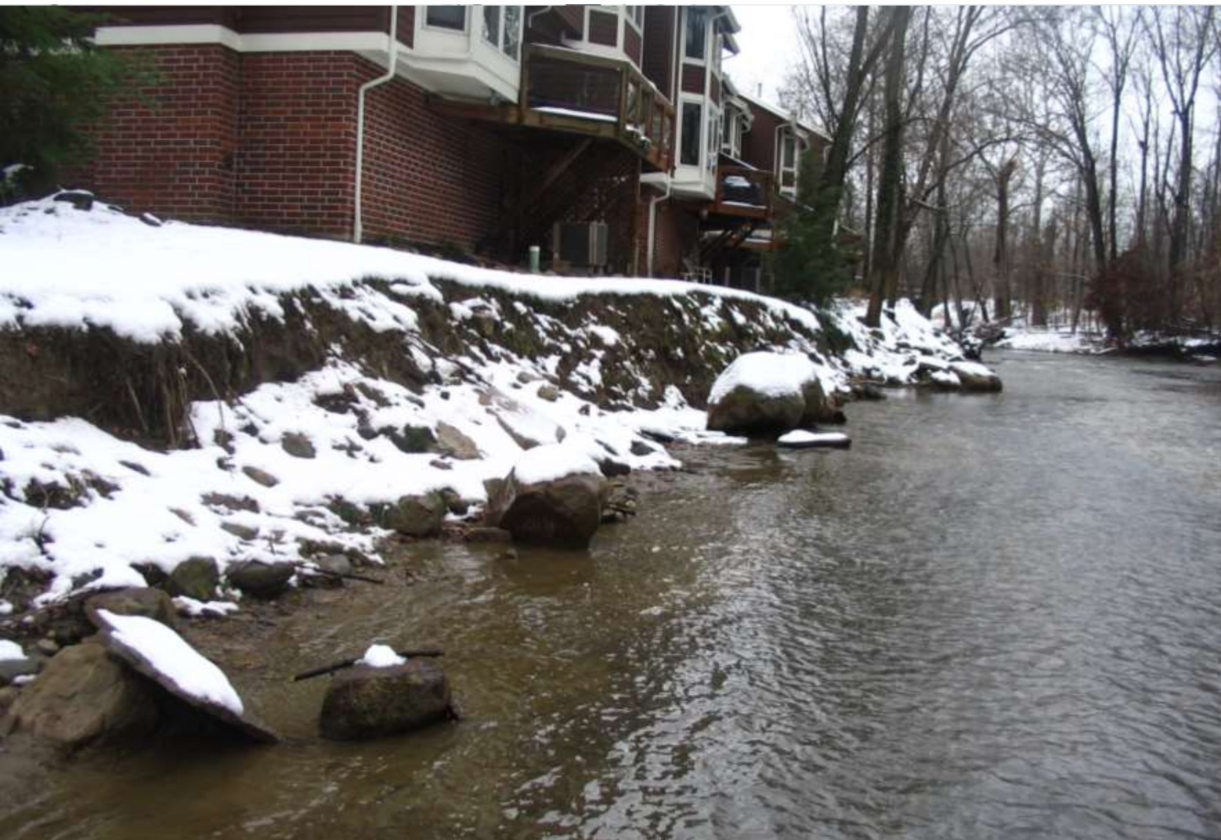
Streambank erosion along Chippewa Creek
