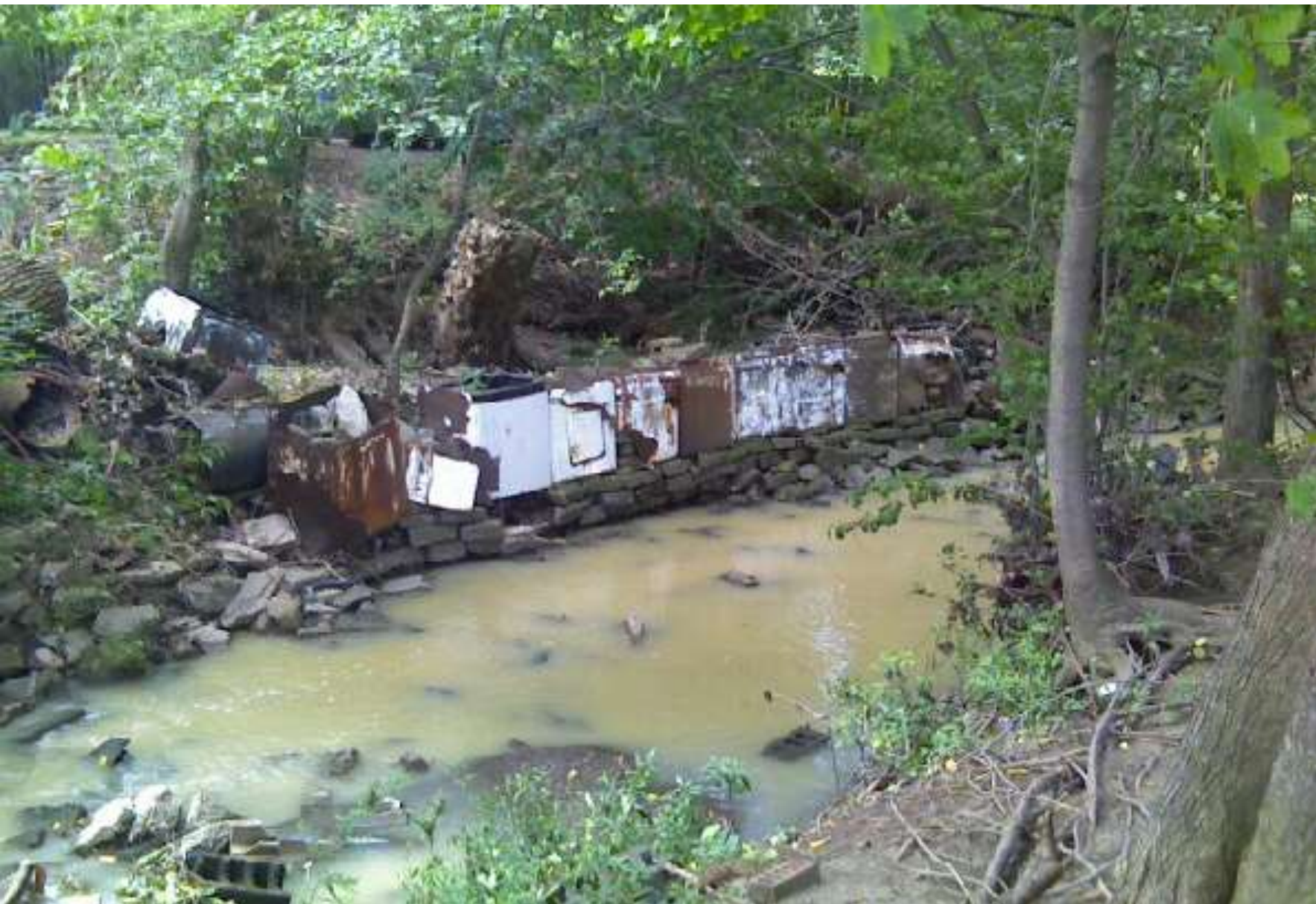
Streambank erosion along Stickney Creek
