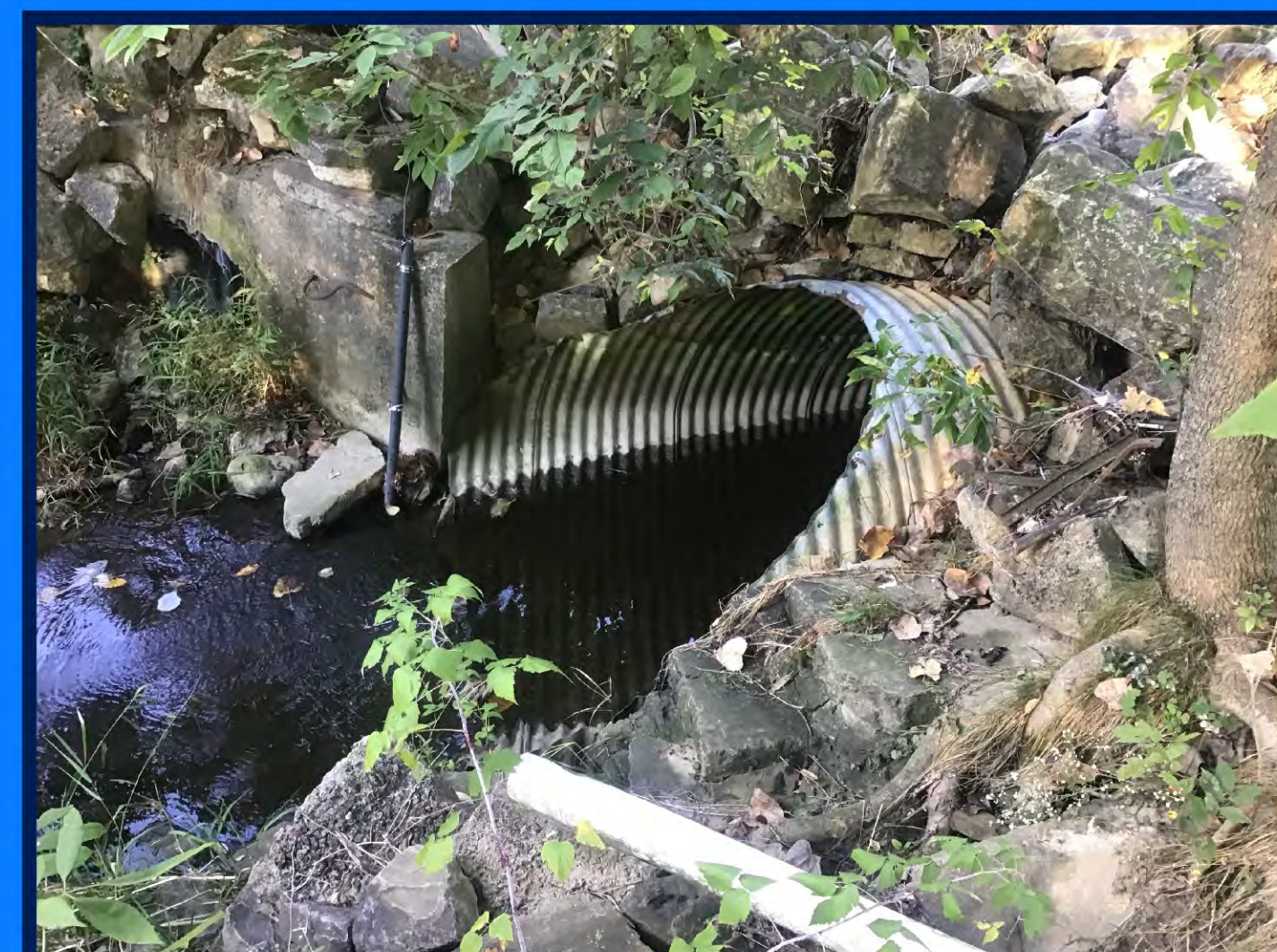
Existing storm sewers that convey flow from Basin CC00231 and local storm sewers, under Echo Lane, to Stream CC00184.
