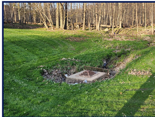
Inlet to the Local Stormwater System at the Eastern End of Echo Lane
