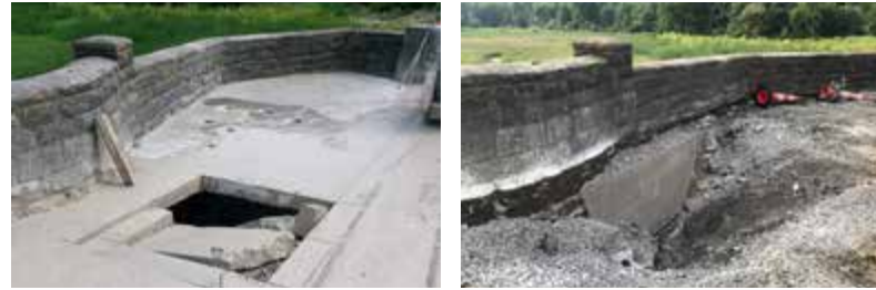
Saw cut and removal of concrete walkway over Horseshoe Lake spillway to investigate detected voids within the dam and spillway structure, July 2021
