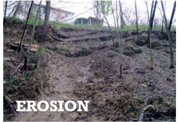
Streambank erosion threatening residences along Big Creek in Parma
